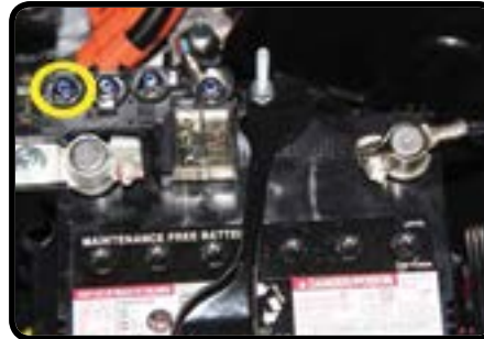
DC to DC Converter Connection
