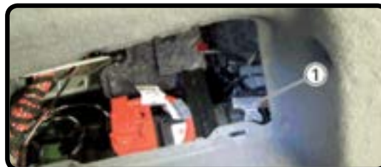
12V Auxiliary Battery Negative Terminal
