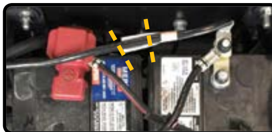
Cut Section Out of the Negative Cable
