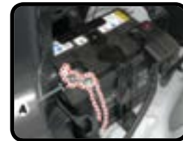
12V Battery In Trunk
