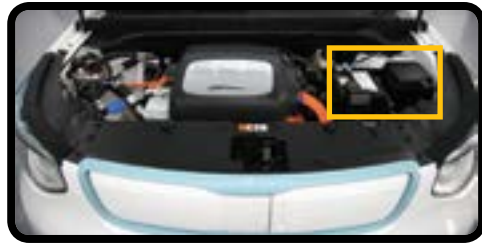
Fuse Box and Battery Location
