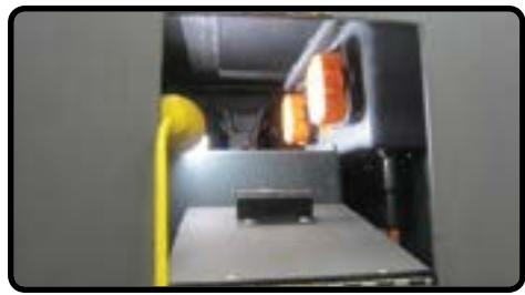
Access Door and MSD's
