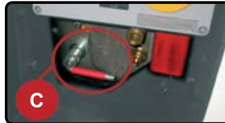
24V Battery Switch
