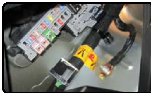
Cut through the positive 12V cable on each side of the tag to remove a section of the cable to ensure the cables cannot inadvertently reconnect.
