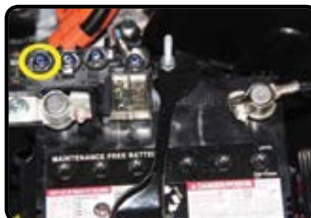
DC to DC Converter Connection
