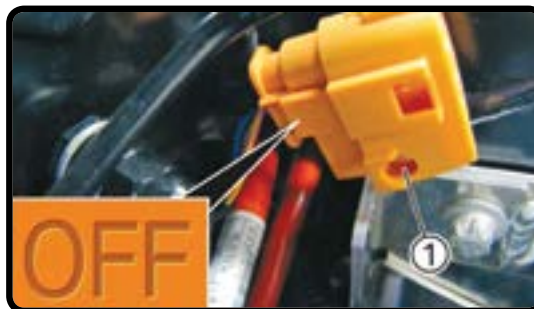
HV Disconnect in OFF Position
