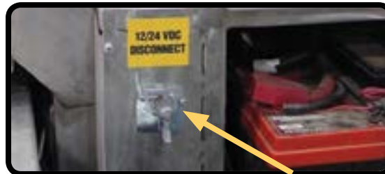
Emergency Disconnect (OFF position)
