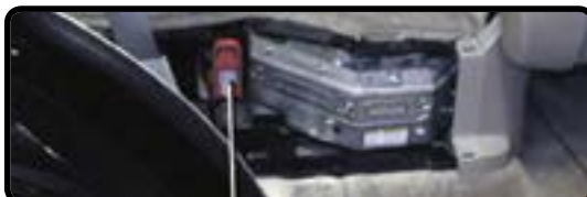
300V Hybrid Battery Manual Disconnect
